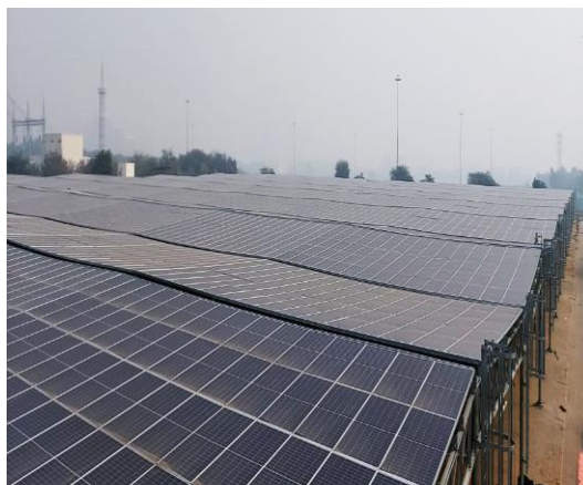
20 MW Solar Carport project, Haryana
