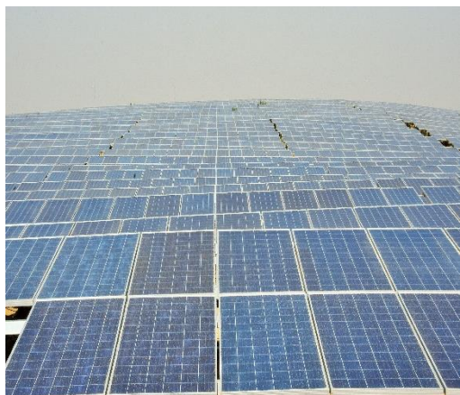
150 MWp Ground Mount Solar Project, Rajasthan
