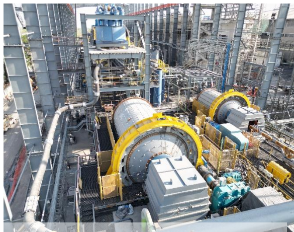
Beneficiation Plant at Dariba, Rajasthan
