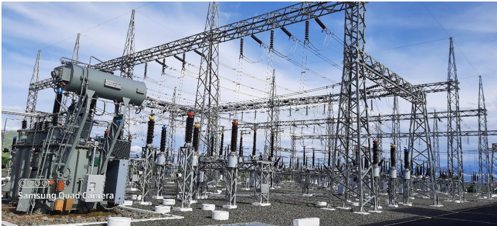
132 kV Air Insulated Substation, Papua New Guinea
