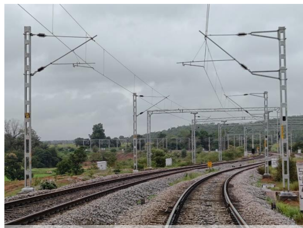
Hubli - Tinaighat Railway Electrification project, Karnataka
