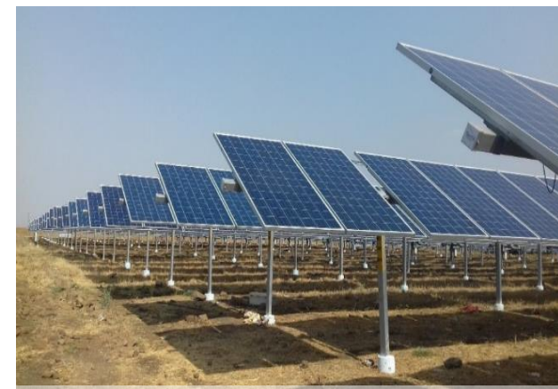
30 MW Tracker Based Installation, Andhra Pradesh
